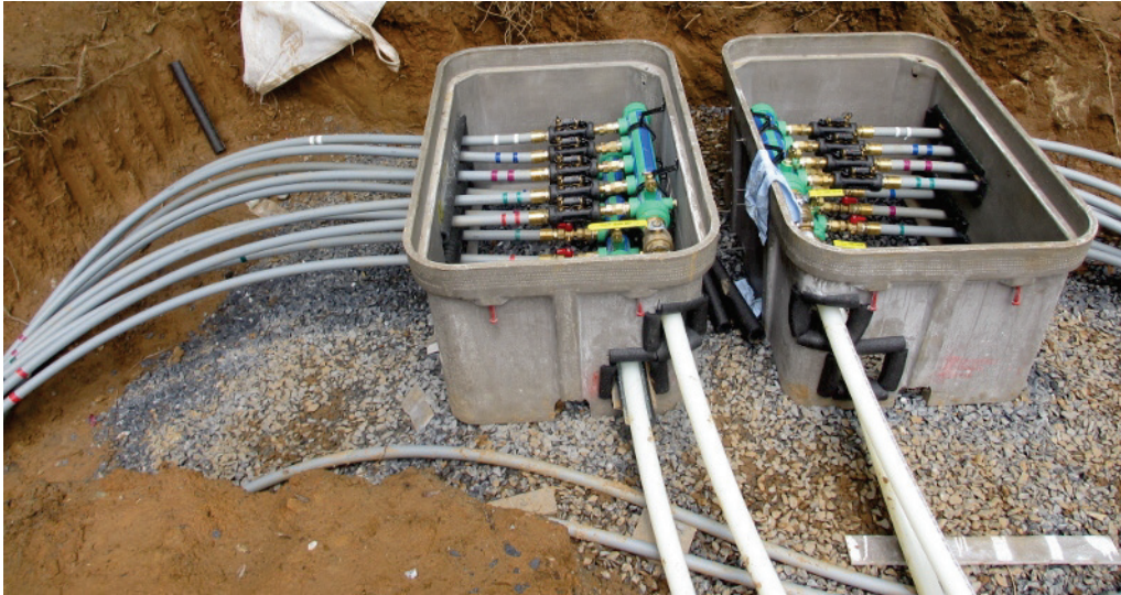
Polypropylene (PP-R) valved manifolds located in small outdoor vaults backfilled with soil
