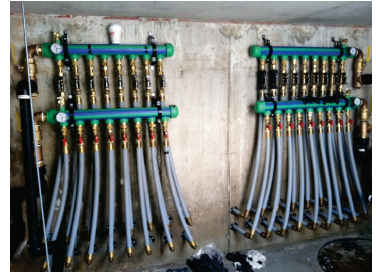
Polypropylene (PP-R) valved manifolds located in concrete vault
